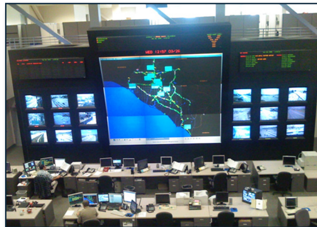
Figure 1. Caltrans District 12 TMC
